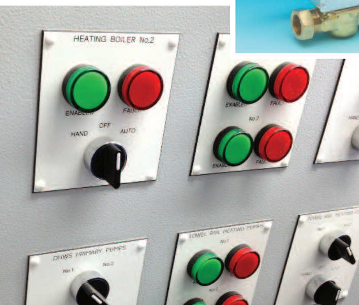
Commercial style control panel
